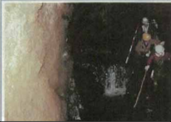
Drop near middle of tunnel, where work crews digging from either end are thought to have met
