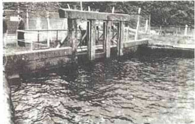
FUKARA Intake Sluice
